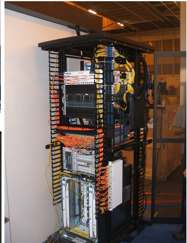
Completed network-demo rack in NASA Exhibit Booth.
