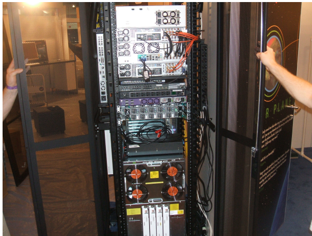
Rear view of full network-demo rack.
