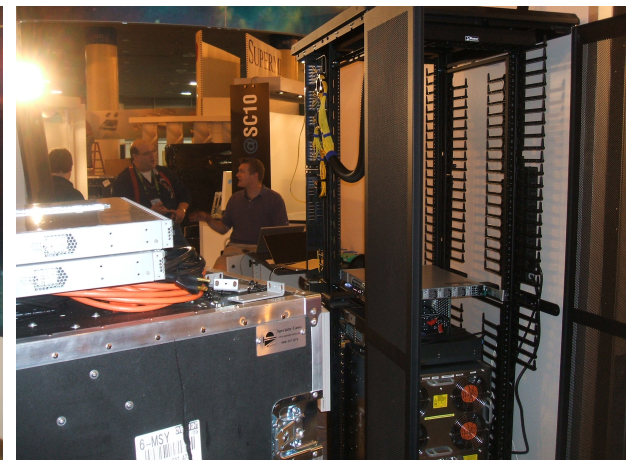
Rear view of the mostly empty network-demo rack.
